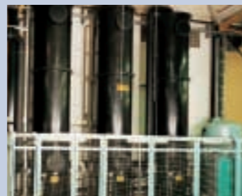
Stripping system at the Stuttgart-Feuerbach plant
