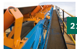
26 Connected conveyor belt
